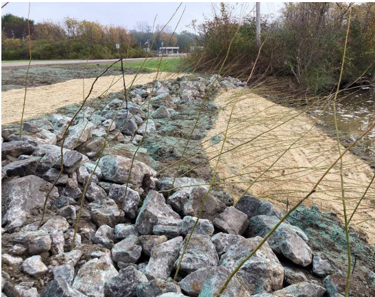
An erosion control project on Ball Creek nears completion (photo taken in October 2021 by Andy Johnson / EcoStrategies)
