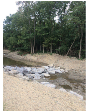
Newly-installed cross channel grade stabilizers and area of new seed/mulch. on lower Bemus Creek.
